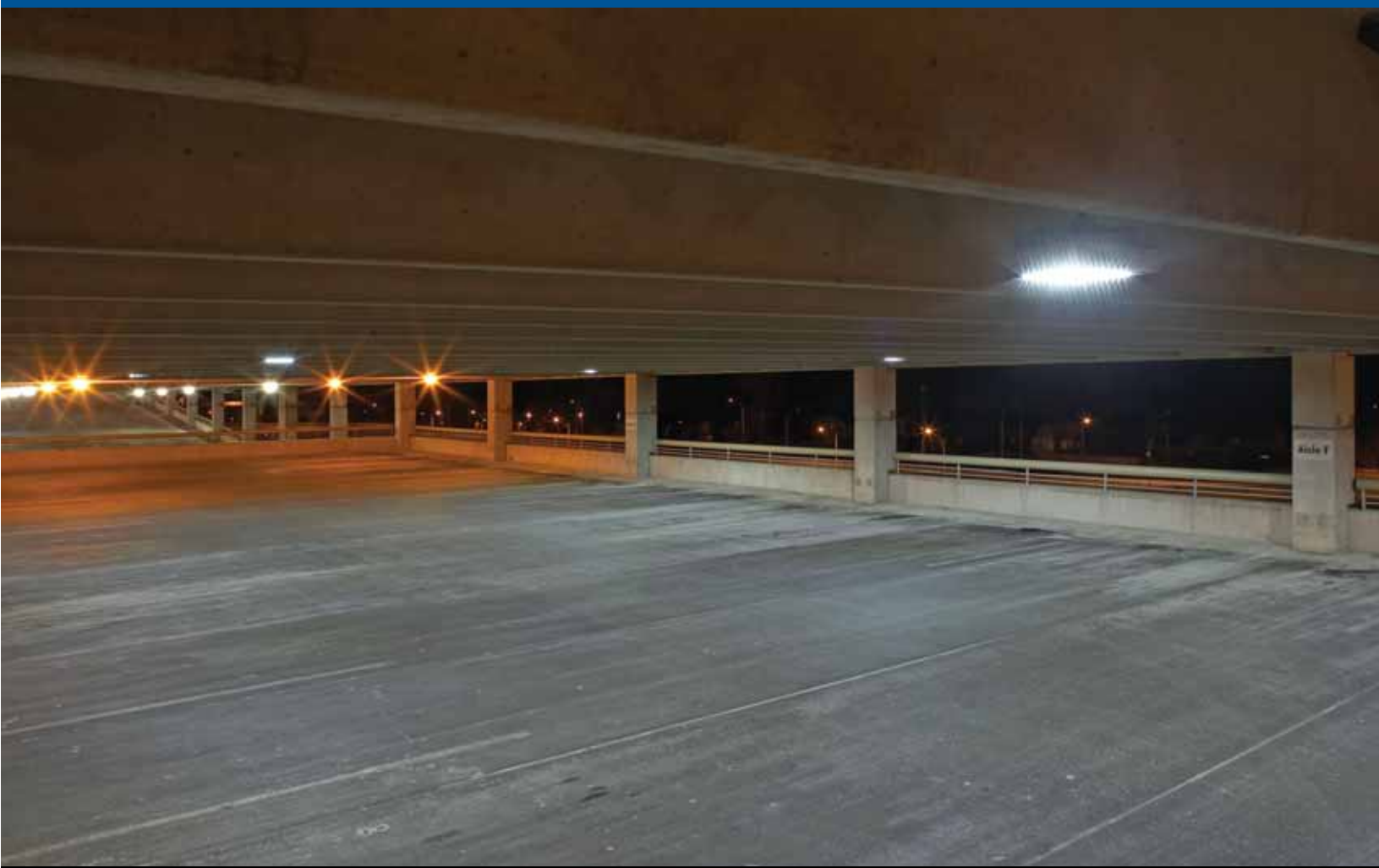
Note the difference in lighting between where High Pressure Sodium and LED lighting is used.
